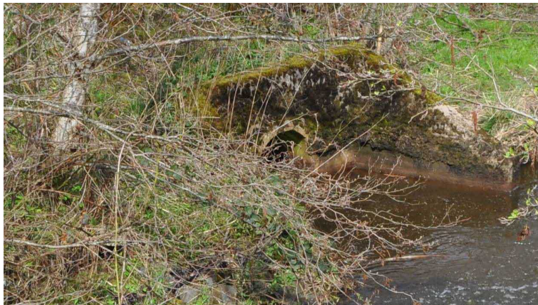
Plate 2 –the South Catchment Outlet where it meets the Bothlin burn. The culvert will be surcharged by approximately 1.5m when the burn is dealing with design storm events.
